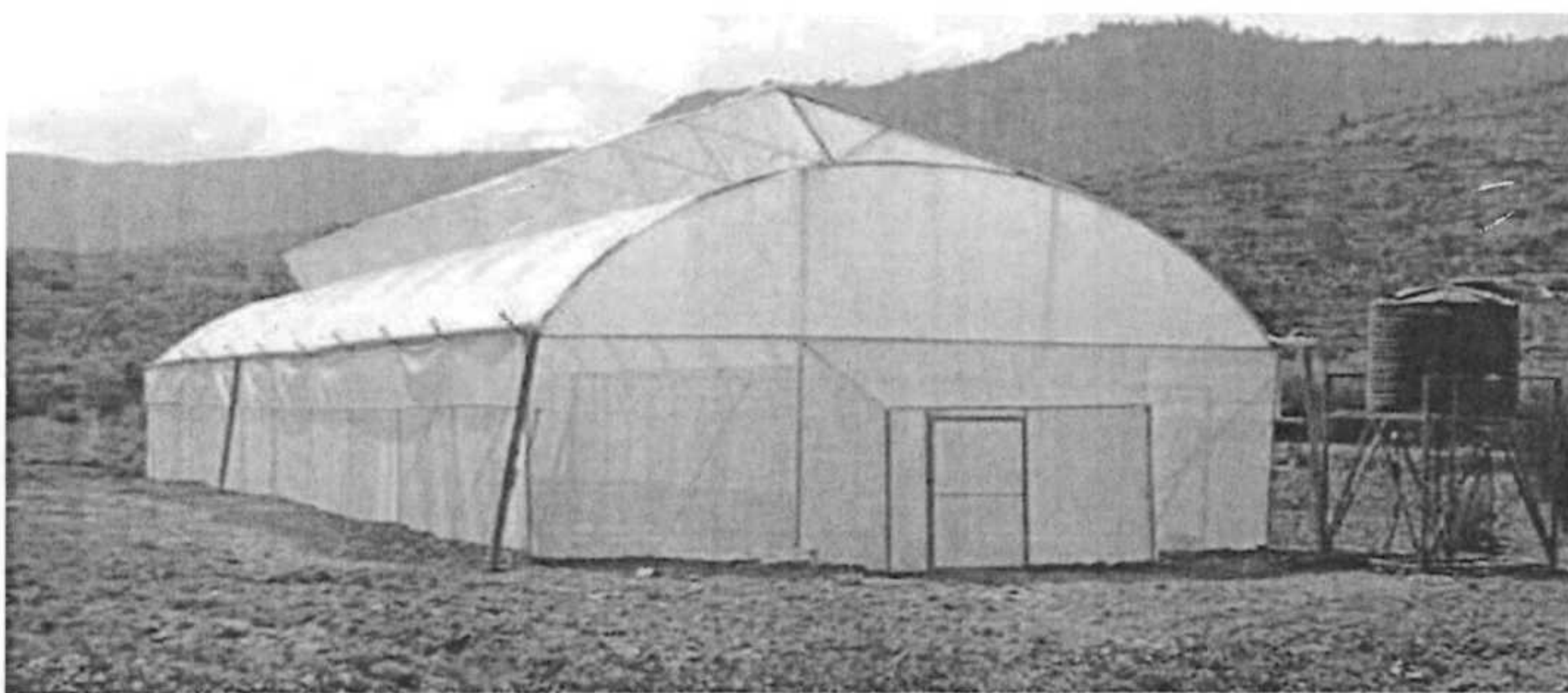
Picture: 8MX30M installed greenhouses
